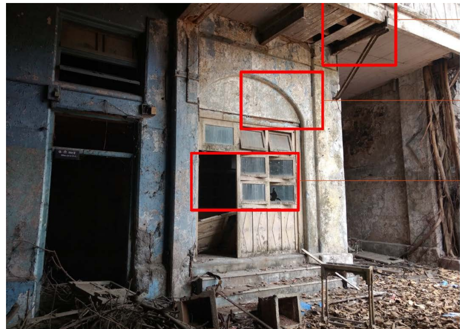
Damaged Flooring Boards
