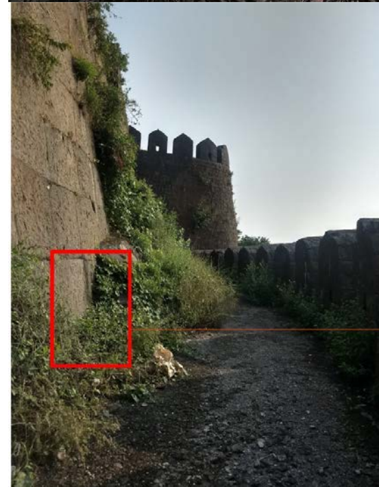
Plants and moss can be seen growing on the walls of the fort
