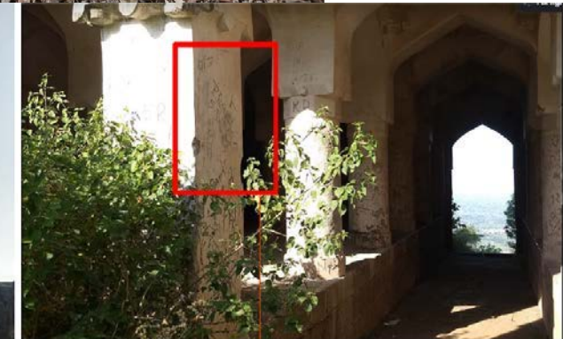
Vandalism by tourist can be seen here. Various names and numbers carved on the wall.
