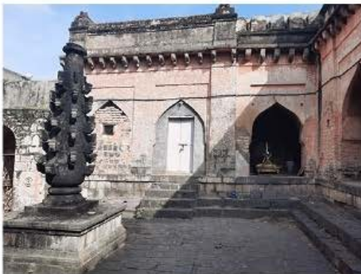
LATER ADDITION OF WALL LIME TERRACE IS LAYERED BY CEMENT WATER PROOFING .
