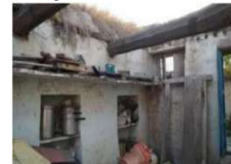
Back part of the house Dilapidated
