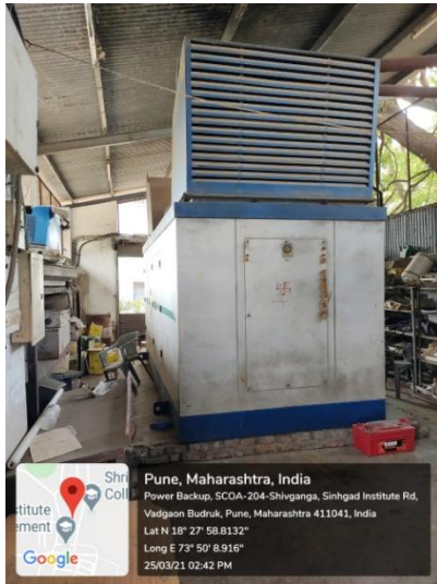
Power Backup system
