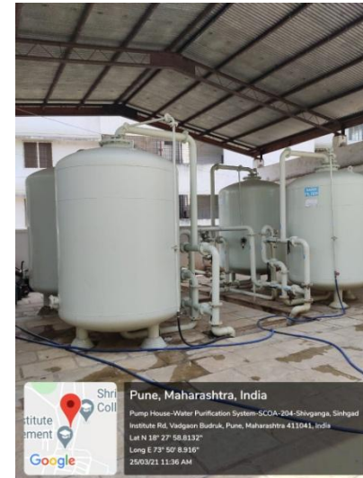
Water Purification system
