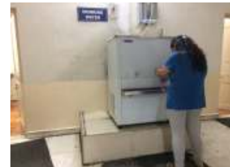
water purification and cooling
